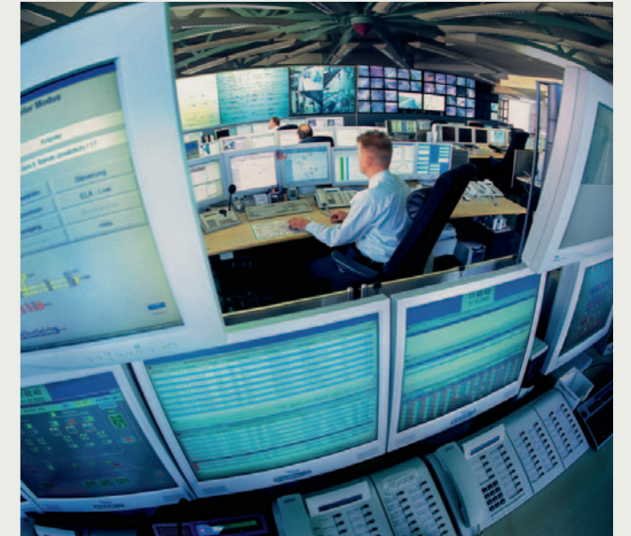
Control and communications systems supplied by Siemens will help facilitate the integration of mass transit and mainline network transport in the Crossrail tunnel.
