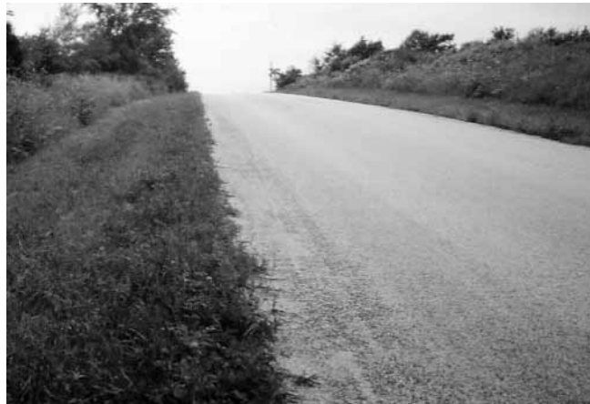
LEFT Road with a good seal and excellent drainage; no maintenance required.
