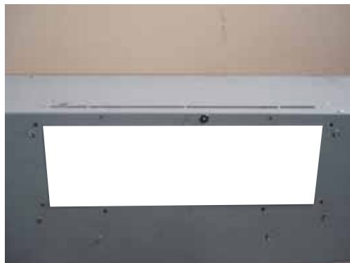
Horizontal Ducting (3-1/4"x10" Rectangular)
