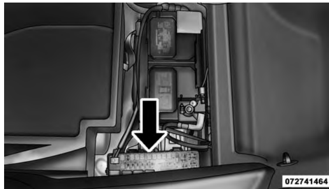
Rear Power Distribution Center
