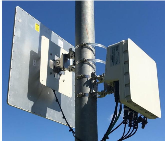
60x60 cm 2 antenna connected to FL58 module with feeders
