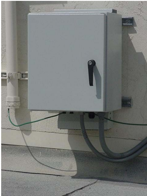
Figure 6: Wall mounted remote unit
