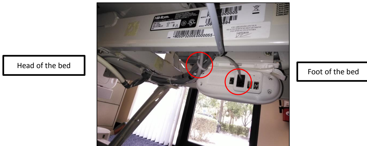
Figure 8. ALP Sensor Cable Routing to Bed Beacon and Cable Tie Holder Placement
