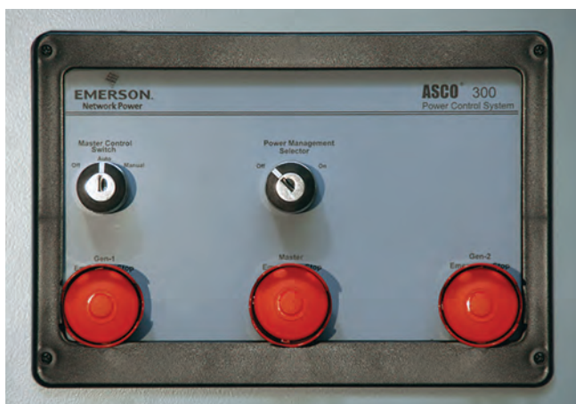
Master Control Panel with Optional Power Management
