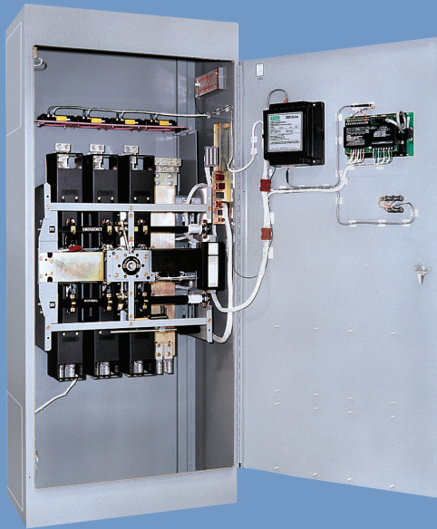
Fig. 1: Three Pole 7000 SERIES Automatic Transfer Switch rated 1600 Amperes (shown with optional front connected terminals and Power Manager).
