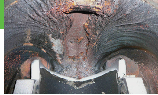
Is damaging erosion like this occurring in your valve?
