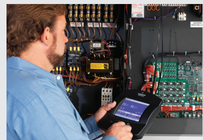
Monitors all key system functions and reports to alarm, if needed. On-board Unit Diary provides a maintenance history to any authorized user.
