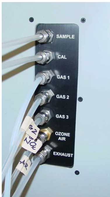
Figure 2-2. MicroCEM Gas Connections
