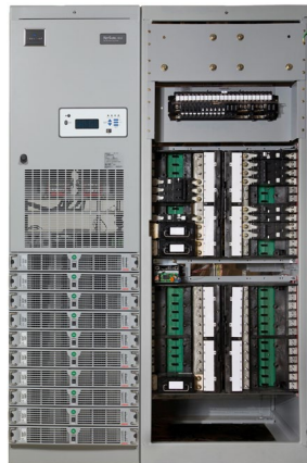
Power Bay with Distribution Bay
