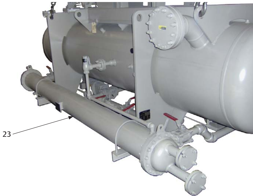
Figure 1-2. Gas Compressor Unit Components (2 of 3)
