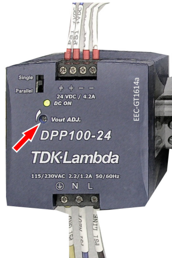
Figure 8. 24VDC Power Supply
