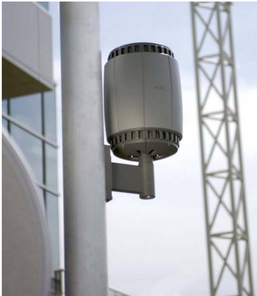
Figure 6: BelAir200 Mounted on a Typical Pole, Ready for Pointing
