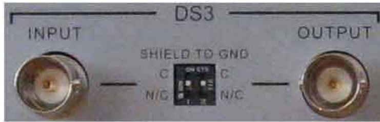
Figure 10 DS3 connectors and grounding switches
