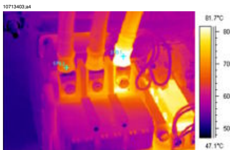
Figure 28.8 An infrared image of indoor electrical equipment (1).
