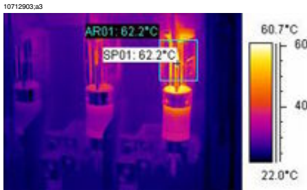
Figure 28.3 An infrared image of a fusebox where the maximum temperature is displayed
