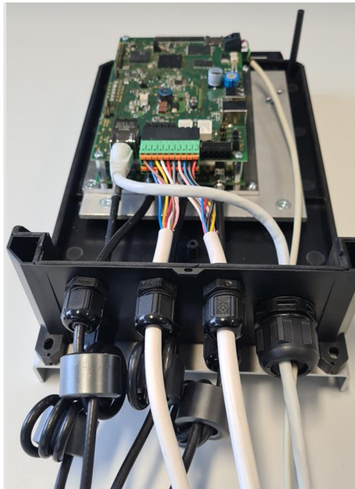
Figure 8: Arrangement of the connecting cables
