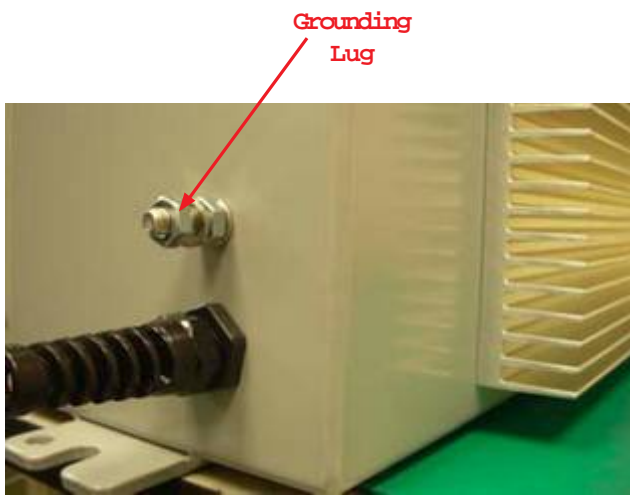
Grounding Lug at Bottom of Wall-mount Chassis
