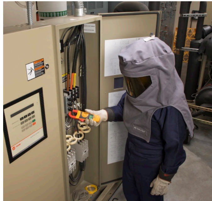
Taking current measurements at a 480 V chiller control, looking for phase imbalances.
