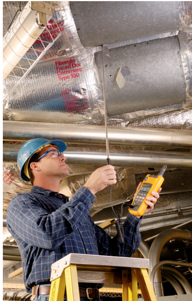
Measuring air velocity in a duct.
