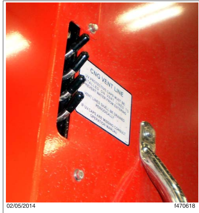
Fig. 21.8, CNG Vent Line Caps
