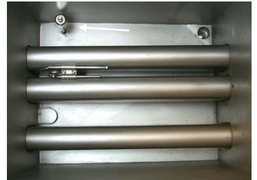
Cook vessel and lower float switch (arrow).
