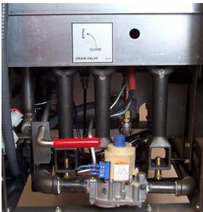
Gas valve and drain handle on spark-module equipped unit.
