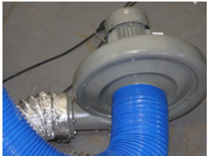
Exhaust fan and tubing
