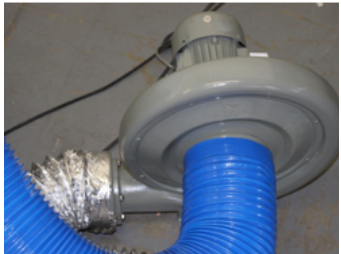
Exhaust Fan and Tubing
