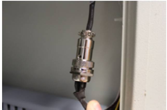
Rotary Attachment Loose Electrical Connection Detail
