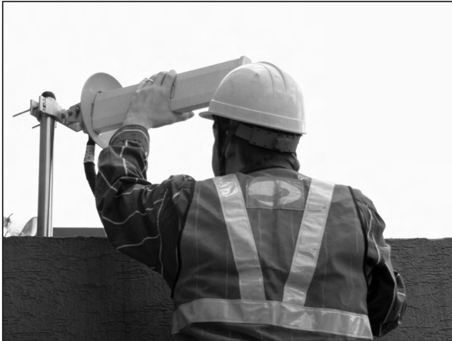
<Figure 4> An installer is directing Donor Antenna to nearby BTS to receive strong input signal.
