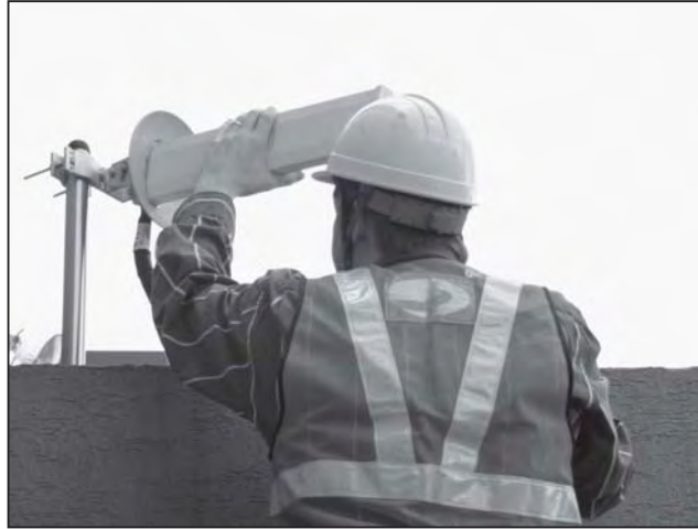
<Figure 4> An installer is directing Donor Antenna to nearby BTS to receive strong input signal.
