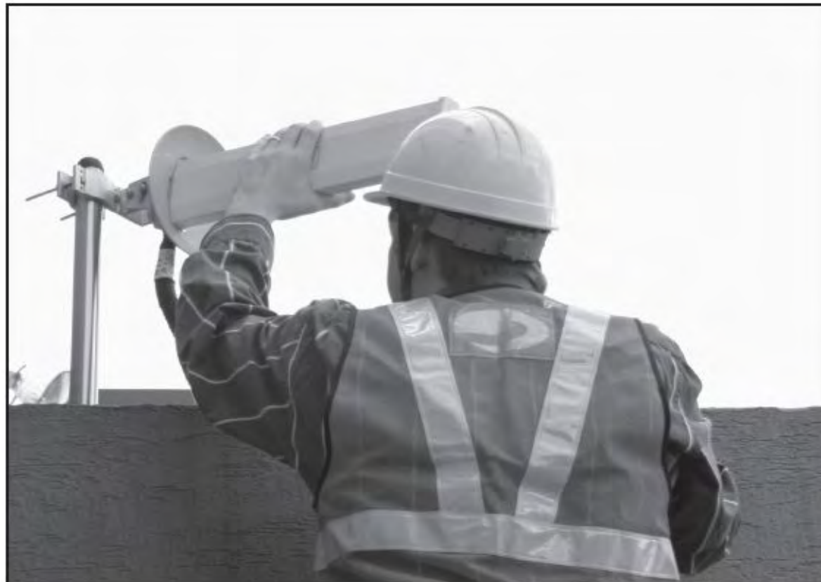
<Figure 4> An installer is directing Donor Antenna to nearby BTS to receive strong input signal.
