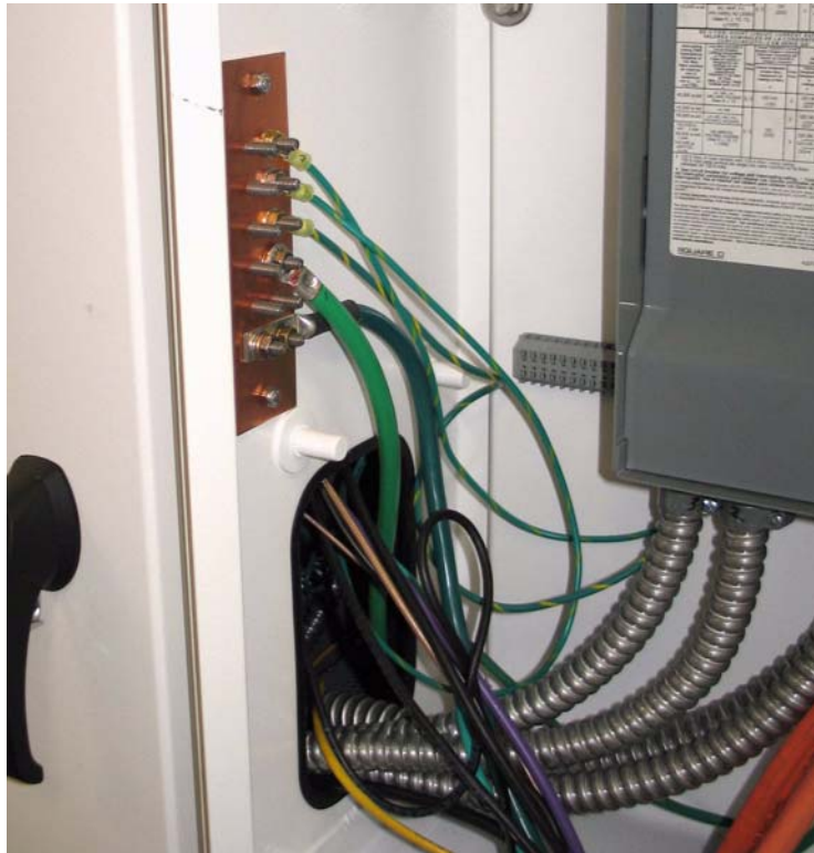
Figure 2-9 System Safety Ground Copper Buss Bar
