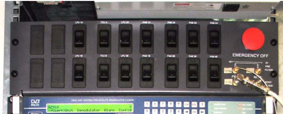
Figure 2-10 Transmitter AC Distribution Panel
