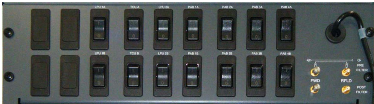
Figure 2-6 Transmitter AC Distribution Panel
