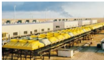
Hassi R' Mel - Algeria Natural Gas Re-injection plant 36 MS5002 Gas Turbines
