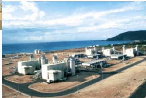
Cape Bon - Tunisia Trans-Med Pipeline Cape Bon to Sicily Head Station 25 MW Gas Turbine Driven Booster Compressors. MS5002 - BCL404/a
