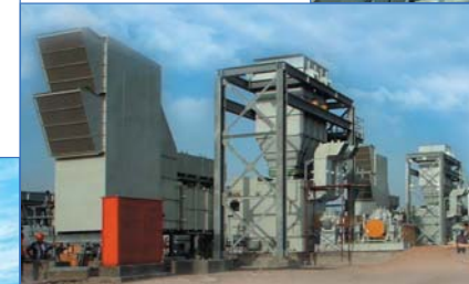
Biskra - Algeria OK1 - SP3bis Station GE10-2
