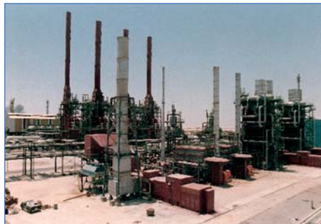
Rhourde Nouis - Algeria MS5001 - MS3001 Gas Turbines and 2BCL 406B Compressors
