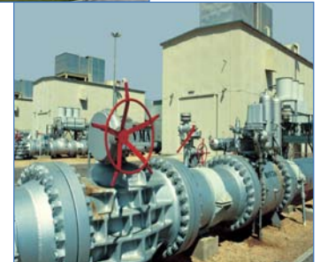
Sbikha - Tunisia PGT 25 - PCL603 Pipeline Compressors
