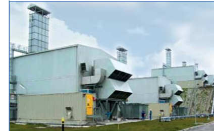
Blue Stream Pipeline Project from Turkey to Russia PGT25 - BCL406/b
