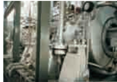
BCL 406/B + BCL 305/C + BCL 305/D compressor driven by MS5002 Gas Turbine installed in Venezuela
