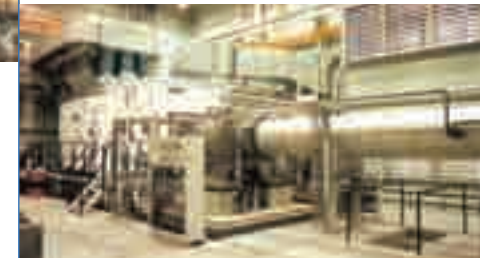
PCL compressor installed in Transcanada pipeline
