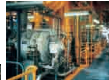
BCL 406/B + BCL 305/C driven by MS5002 Gas Turbine installed on Nkossa platform - Congo
