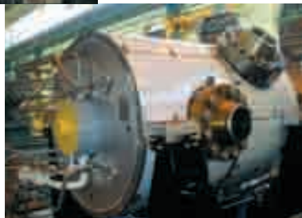
Storage to Pipeline Compressor Gazprom
