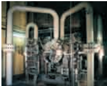
GDF Chemery Gas Storage
