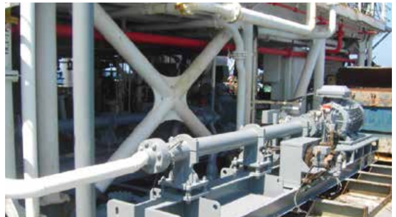
FPU crude oil transfer (Gulf of Mexico)
