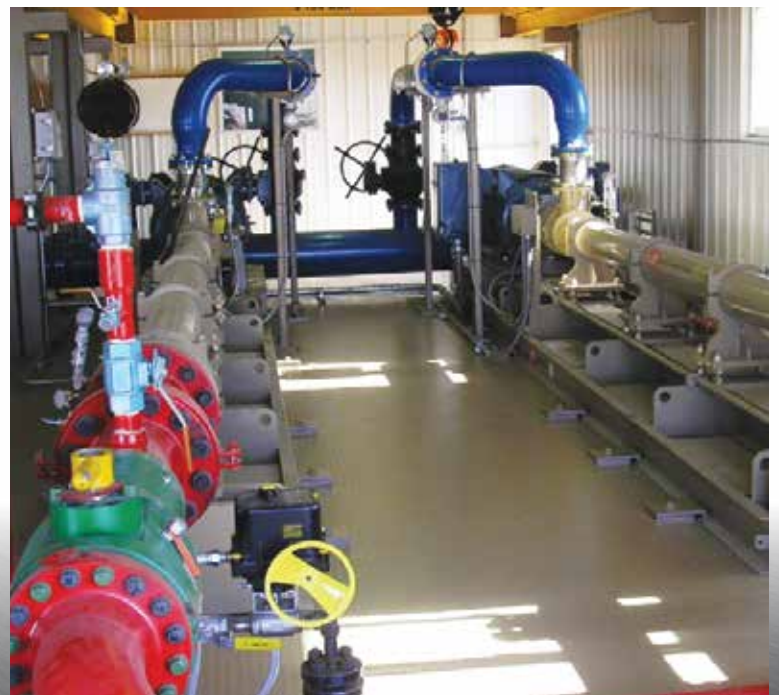
Two of three FM1000s inside custom fabricated enclosure
