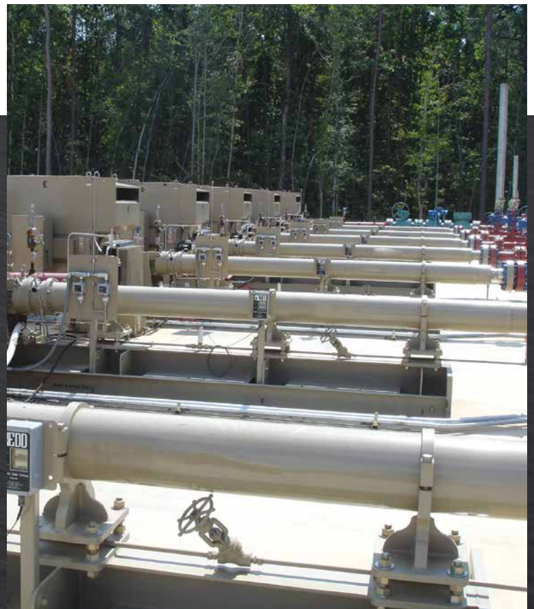
CO 2 pipeline booster (North America)
