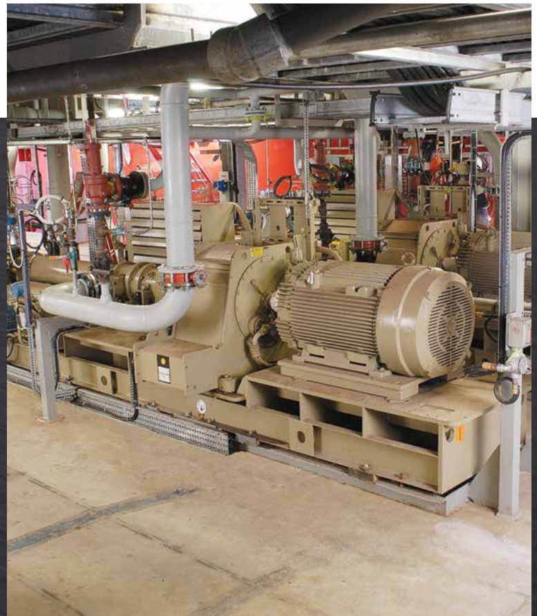
FPU crude oil transfer (South America)
