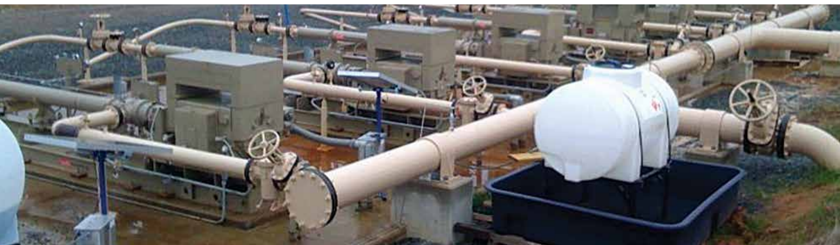
Water transfer installation (North America)
