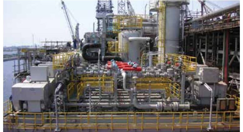
FPSO treated sea water injection (Africa)
