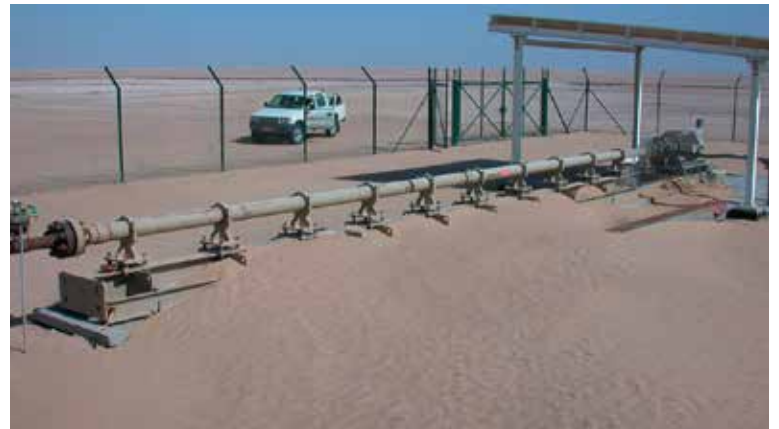
Water injection (Middle East)
