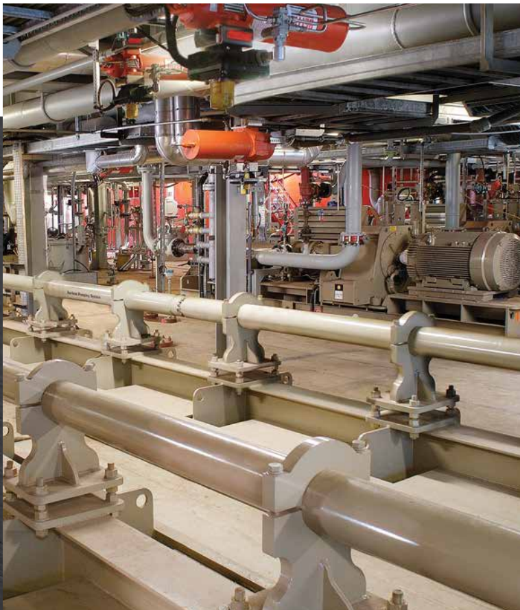
FPU water injection (South America)
