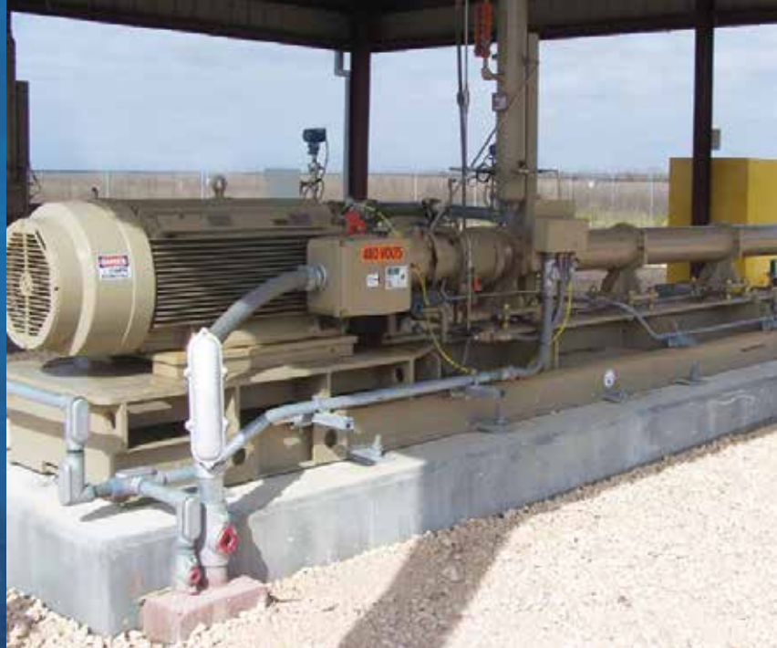
Ethane pipeline booster (North America)
