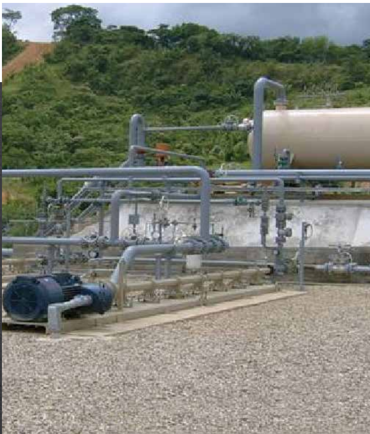
Crude oil and Produced Water Injection (South America)
