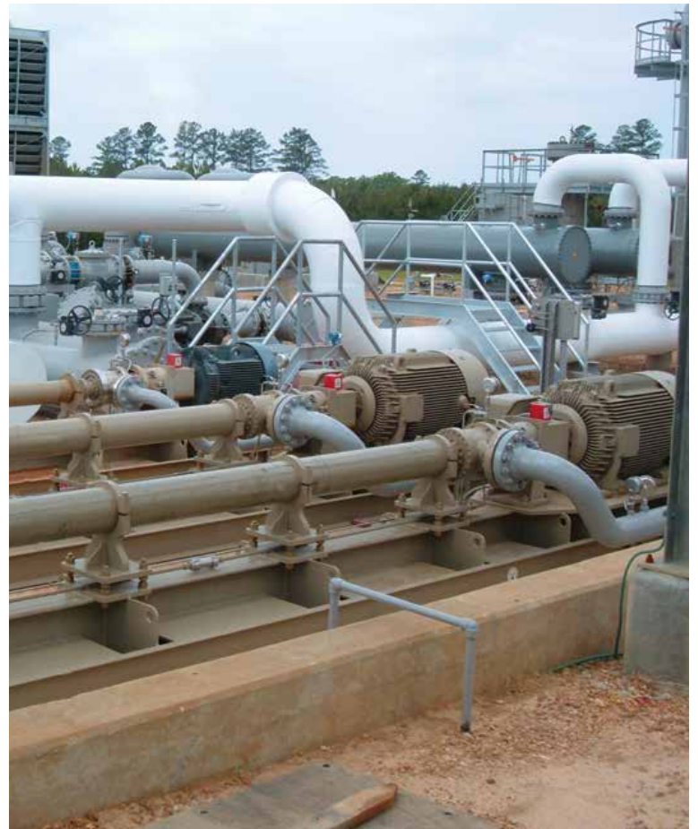
CO 2 pipeline booster (North America)
