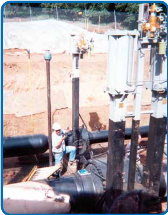
Figure 11 - Installation of Becker Below Ground Regulators (Prior to Backfill) A large natural gas transmission/distribution company based in Southern California installed Becker Below Ground Ball Valve Regulators to achieve maximum noise attenuation, minimal maintenance, and optimum cost effectiveness. The Below Ground Regulator can provide up to 37 dBA additional noise attenuation with minimal additional cost. Two different size Below Ground Ball Valve Regulators are shown here. 16" Bore Below Ground Regulators are shown in background, while 30" bore Below Ground Ball Valve Regulators are shown in foreground. The Below Ground Ball Valve Regulators are shown during installation, prior to backfill of the regulator station.
