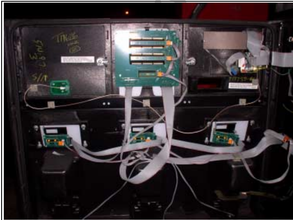
Figure 25: Cable Properly Dressed from Antenna to Card Reader
