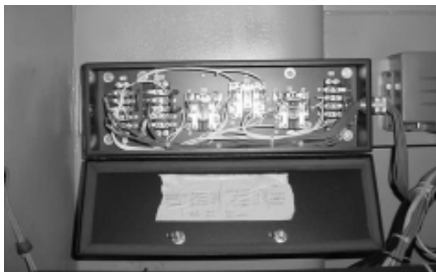
Figure 1.3-5 Headlight Control Module
