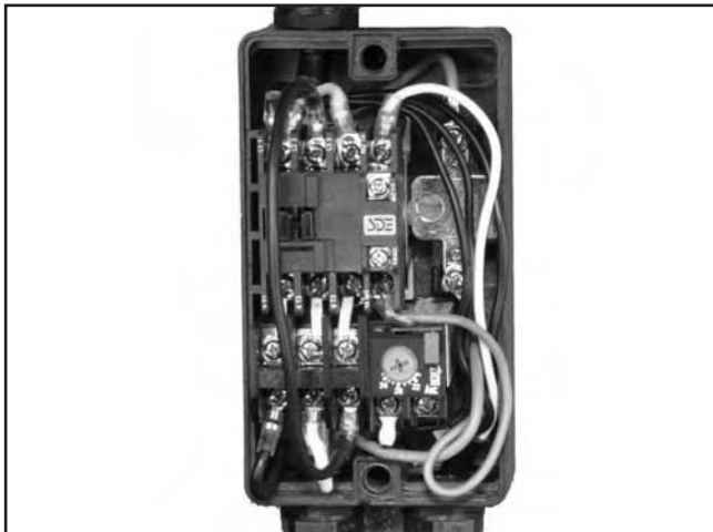
Figure 4. 220V Magnetic Switch
