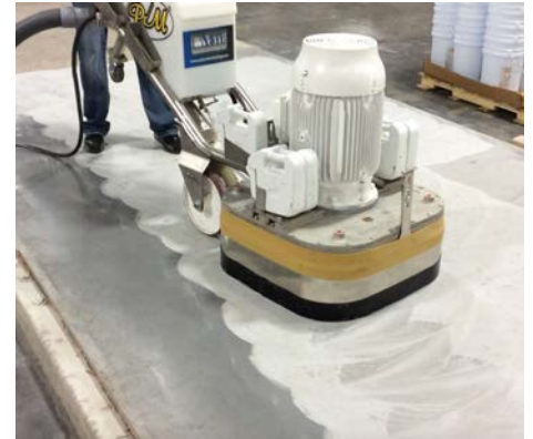
From Concrete Prep to Polish – P/M Machines can tackle any sized project on any flooring surface!
