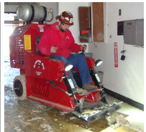
BRB-2800 ride-on floor scraper easily removes VCT during an office renovation project. Hydraulic steering and a zero-turn radius enabled the highly maneuverable BRB-2800 to be used in tight areas.
