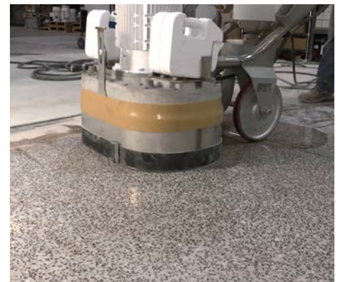
Restoration of a Terrazzo floor using the STI-2807 Machine, TPS Diamond System, and Grout Pans
