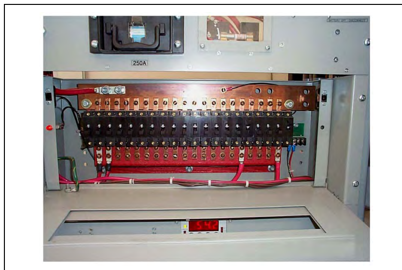
Figure 3-17: -48 Volt Breaker Distribution Panel of the DC Power Supply - Red Wire
