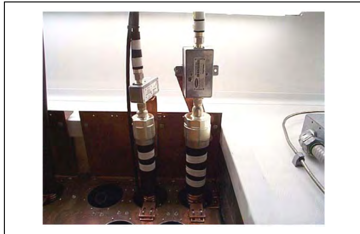
Figure 3-22: Dual Antenna PolyPhasers (Surge Protectors)
