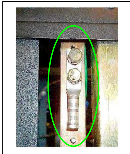
Figure 3-20: Single Point Ground That is Found on Each Rack
