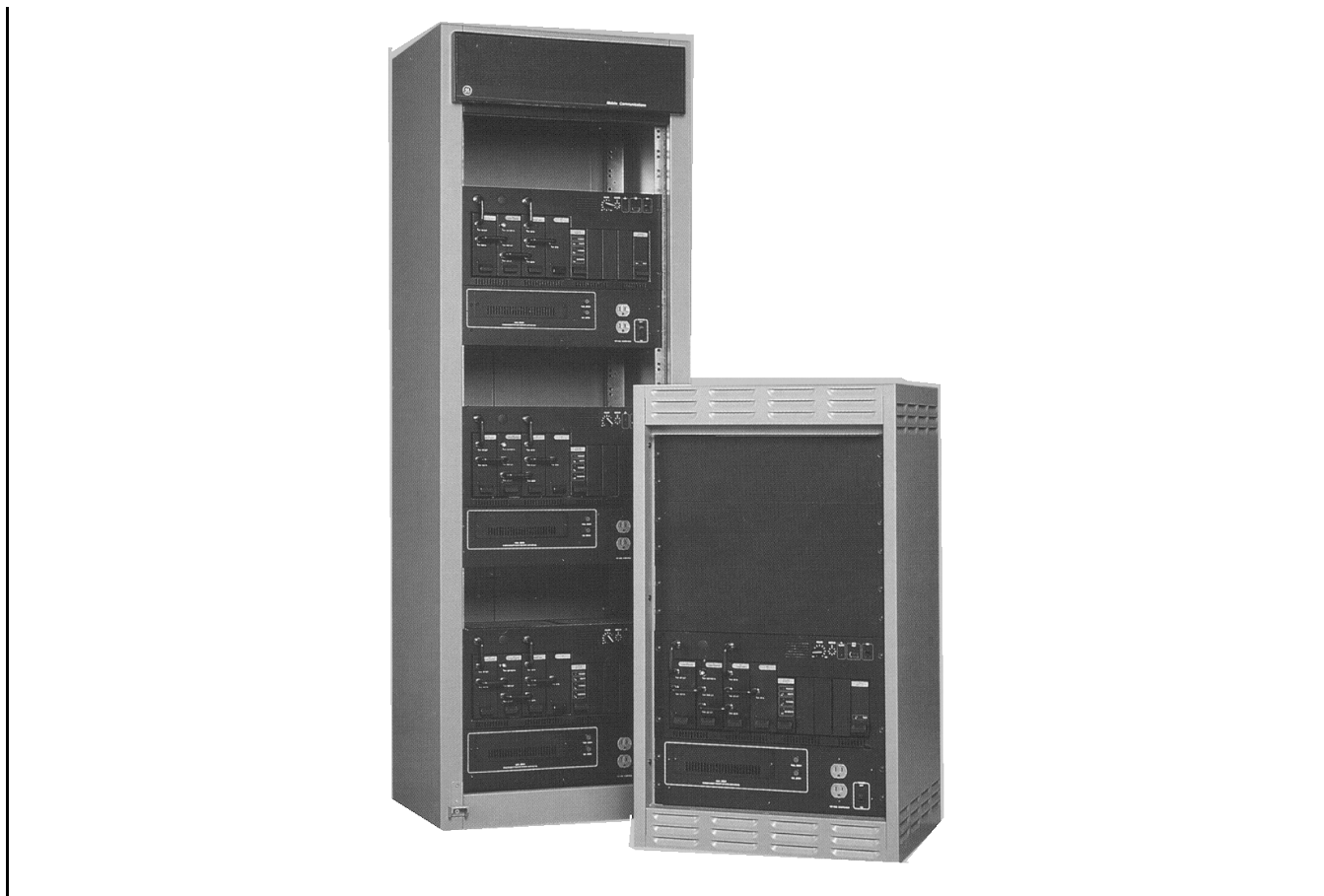
Figure 1 - Typical 37-inch MASTR III Stations
