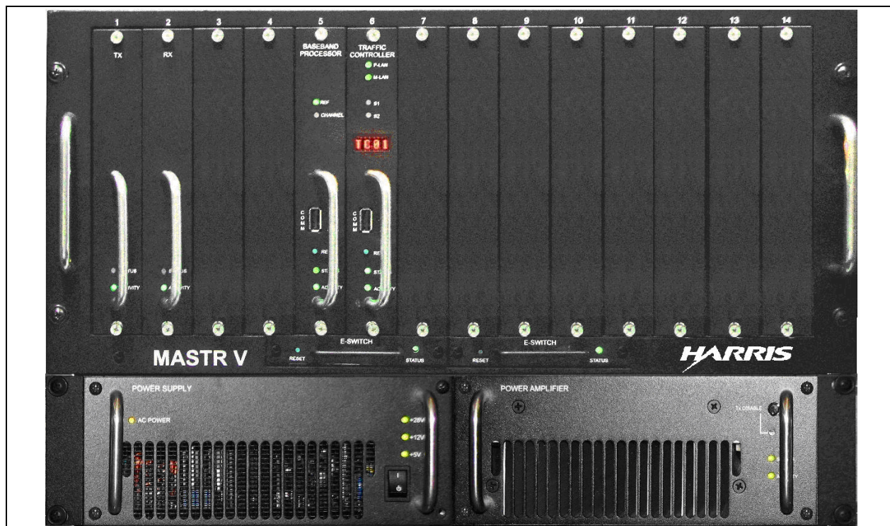
Figure 3-1: MASTR V Multi-Channel Base Station Shelf Equipped with One (1) RF Channel
