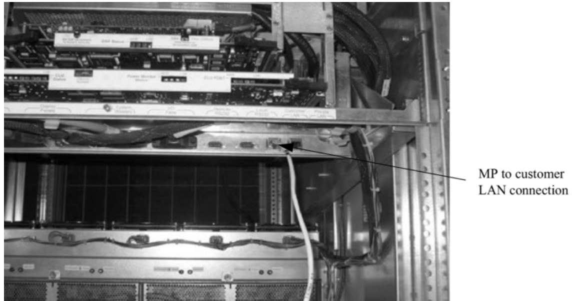
Figure 39 MP LAN Connection Location
