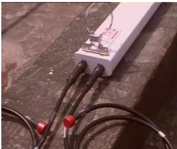
Figure 3-7 Connection between directional antenna and jumper and jumper connector after treatment
