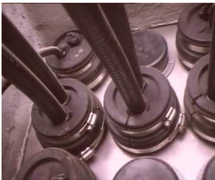
Figure 3-38 Encapsulation treatment of the feeder window after feeder enters the equipment room
