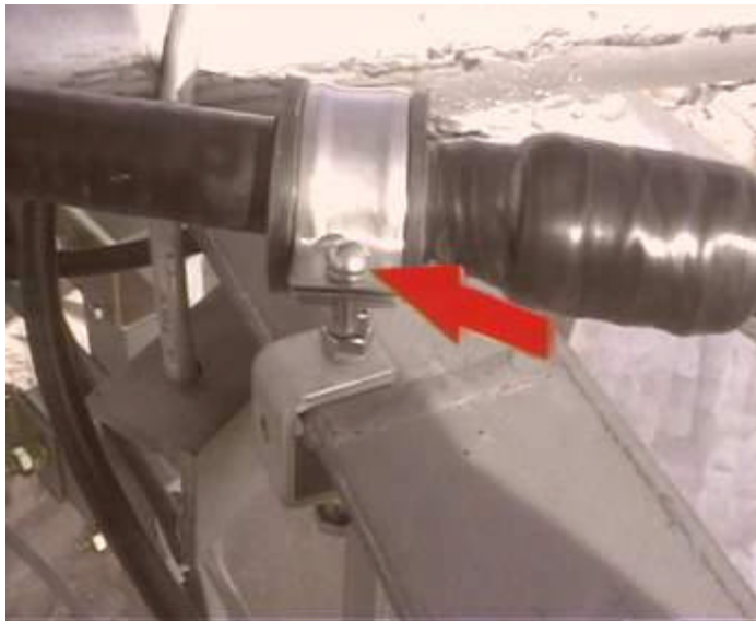
Figure 3-35 Feeder upper end fixed on tower
