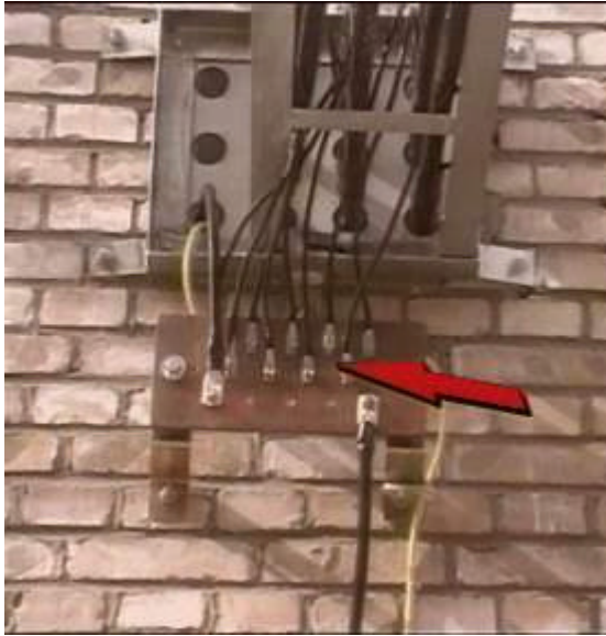
Figure 6-70 Grounding when the feeder does not enter the equipment room (grounding bar available)
