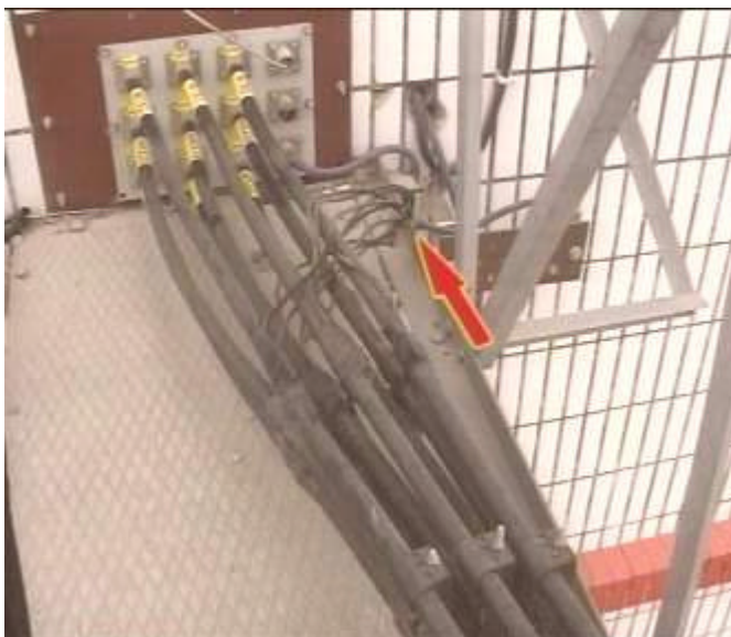
Figure 6-71 Grounding when the feeder does not enter the equipment room (grounding bar unavailable)
