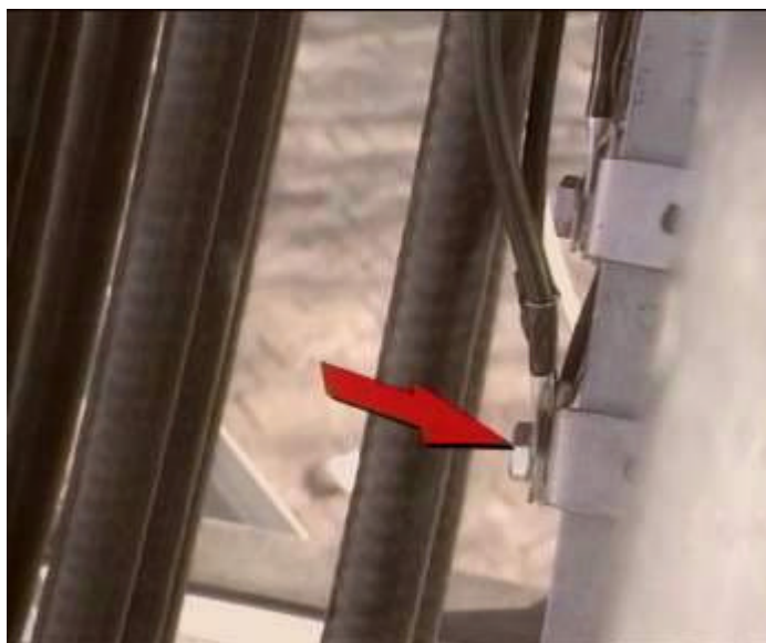
Figure 6-69 Connecting the grounding cable of the feeder grounding clip to the steel plate of the tower
