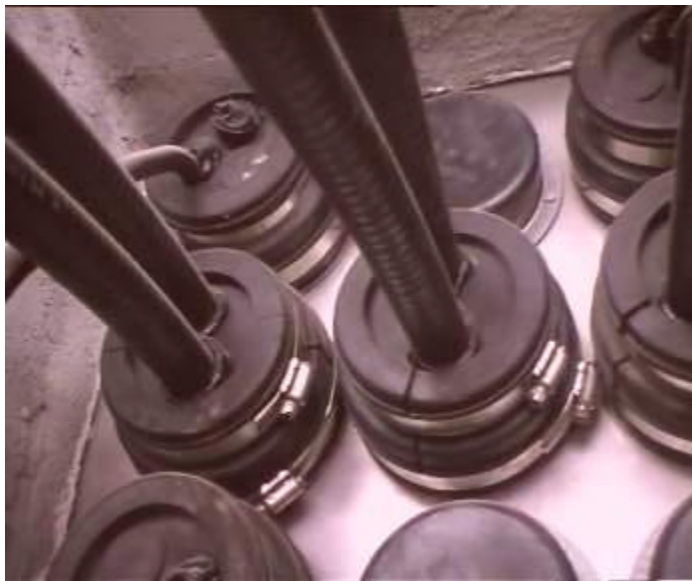
Figure 3-38 Encapsulation treatment of the feeder window after feeder enters the equipment room
