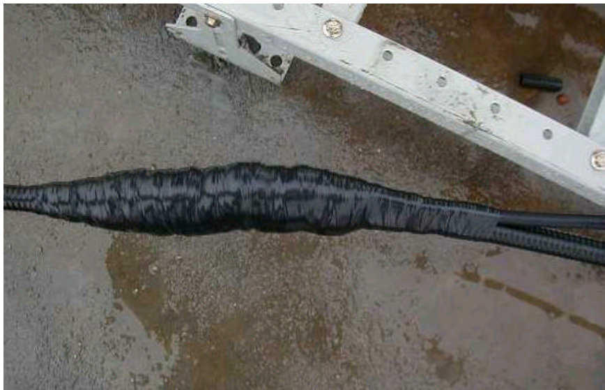
Figure D-4 Wrapping lightning protection grounding clip with three layers of tapes
