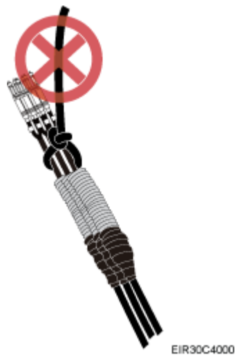
Figure 7-8 Incorrect binding method
