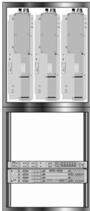
Indoor centralized installation, -48 V power supply
