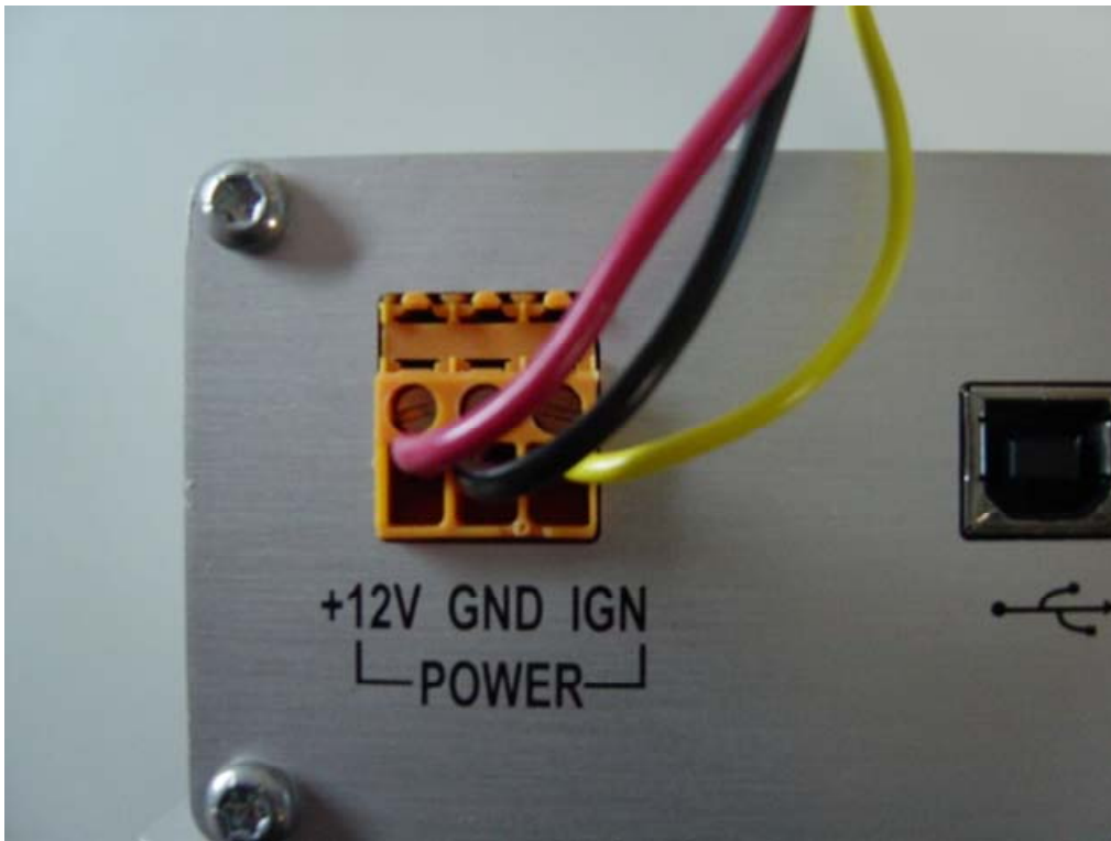
Figure 13 Power Cable Connection to TMG
